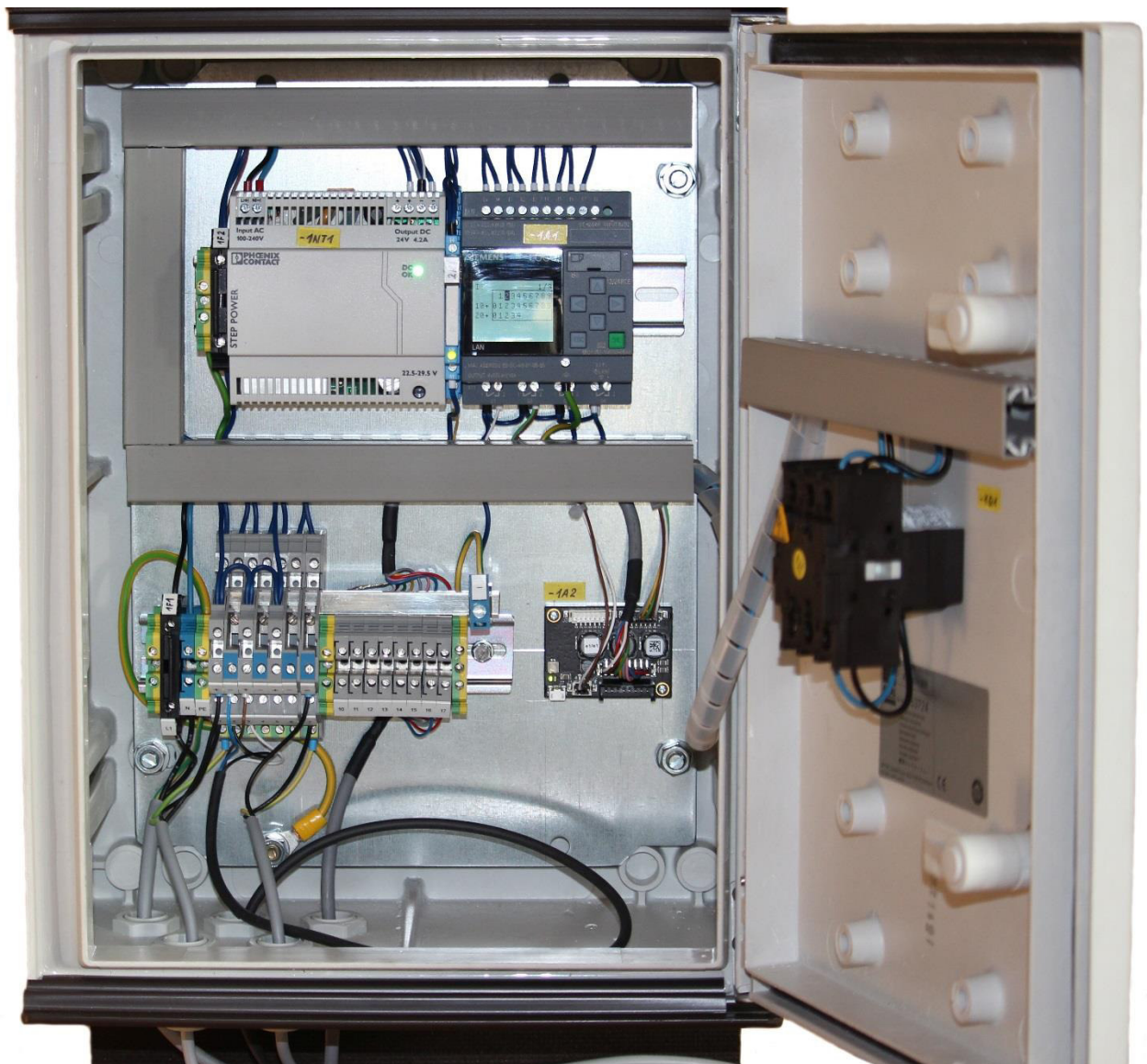
Cabinet with Siemens Logo! and controller for brushless DC gear motor
